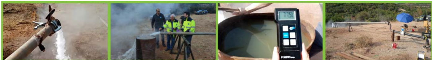
Well testing at the Sidirokastro geothermal field in Serres, Greece (source: HSGME)
