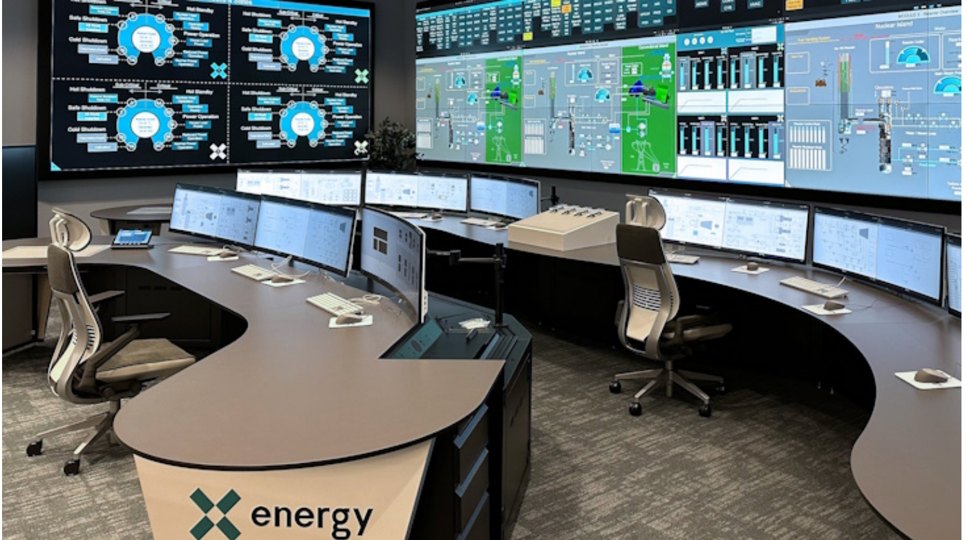
A control room simulator is the centrepiece of the state-of-the-art facility (X-energy)
